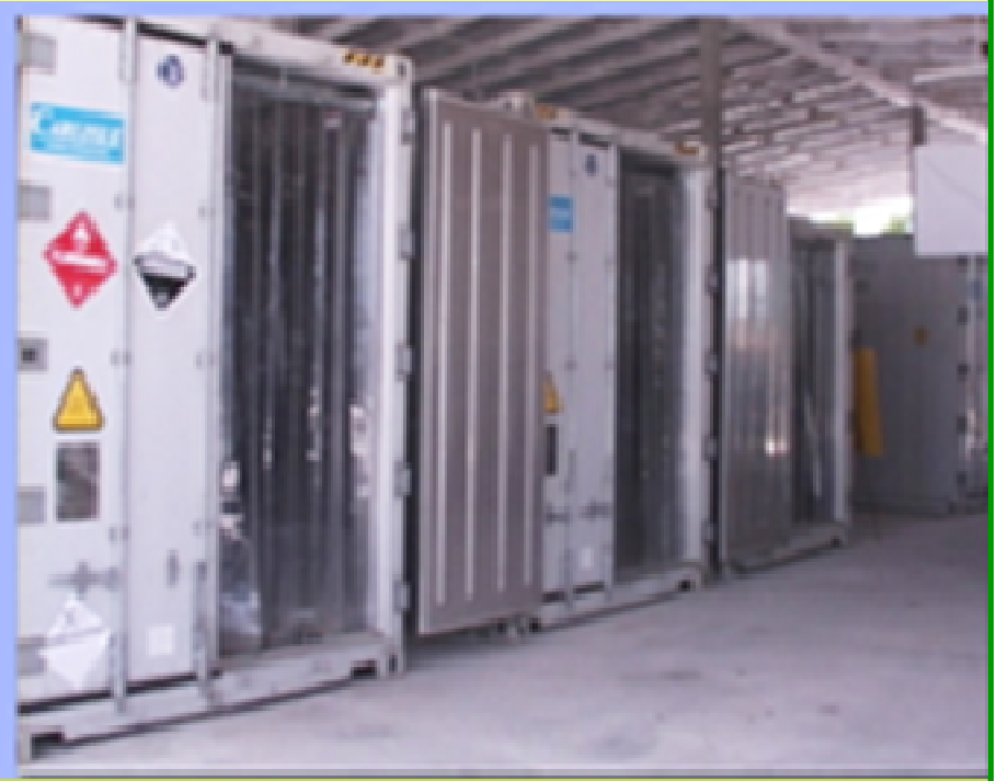
Cold Storage Facility at Chiddi Jagan International Airport
